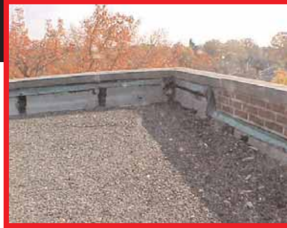
An illustration of a roof that runs up the back of a parapet wall.
