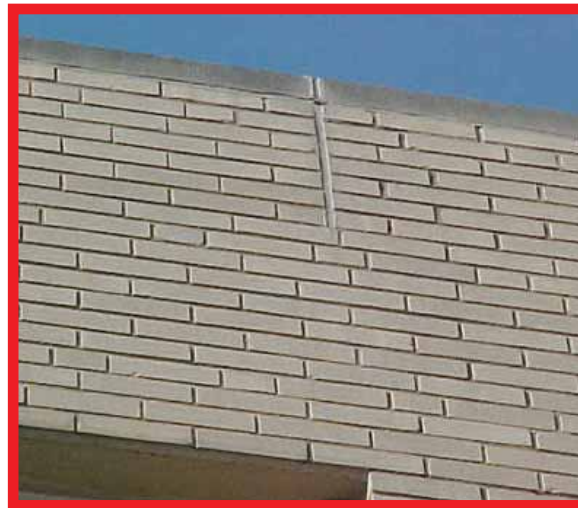
Incomplete Expansion Joints
