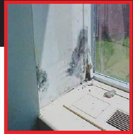
Water-damaged window soffits, jambes and sills.
