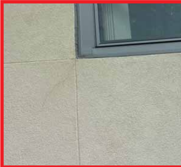
Cracking through EIFS lamina.
